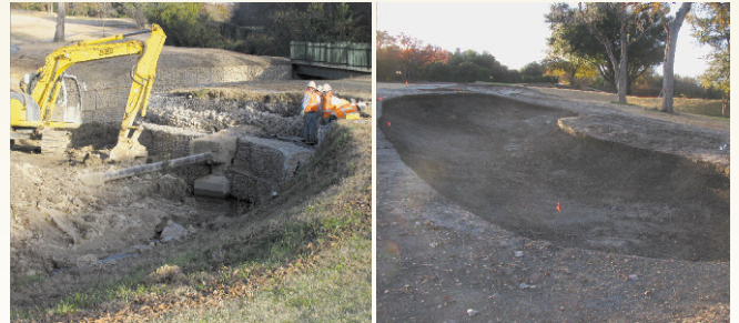
Pictured above are the drain line installation on #7, new irrigation controllers on #13, the right green side bunker on #6, the new gabion erosion control on #6 and the first right side bunker on #8.
